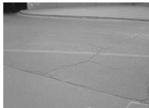
(c) 裂缝病害(块裂)
